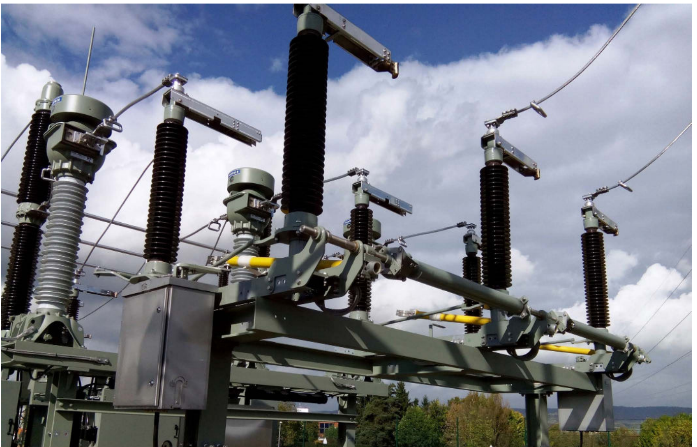
Three-pin, horizontal disconnecter 123 kV at a substation in Hofheim
