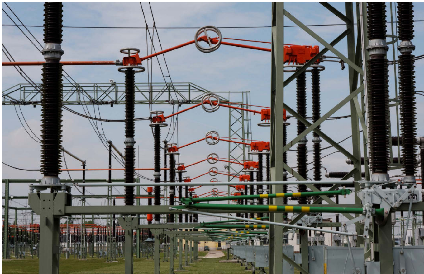
High-voltage switches installed in a substation
