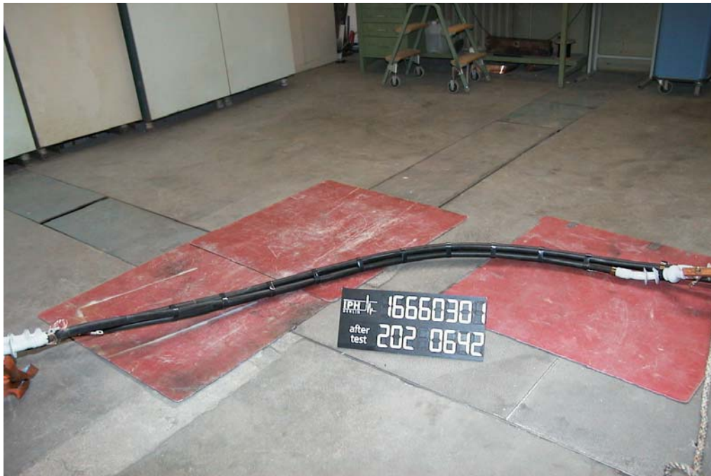
Figure 6: View of test objects after the dynamic short-circuit test
